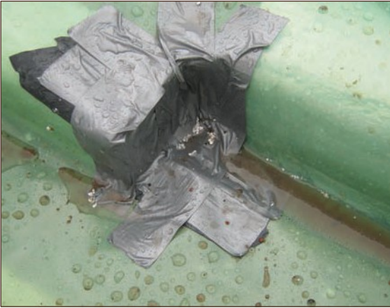
Figure A4.69 Attempt at corner detailing using non-proprietary duct tape (courtesy Smith Grant)
