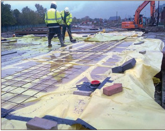
Figure A4.67 Traffic over mesh resulted in several punctures, in addition most joints were found to be poorly constructed. Taped joints are difficult to construct in adverse weather (courtesy Smith Grant)
