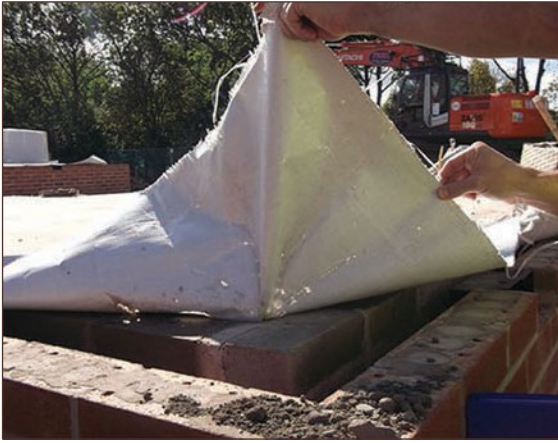
Figure A4.49 Lifted gas membrane at corner position. Light penetrating through confirms damage to aluminium internal core layer (courtesy NHBC)
