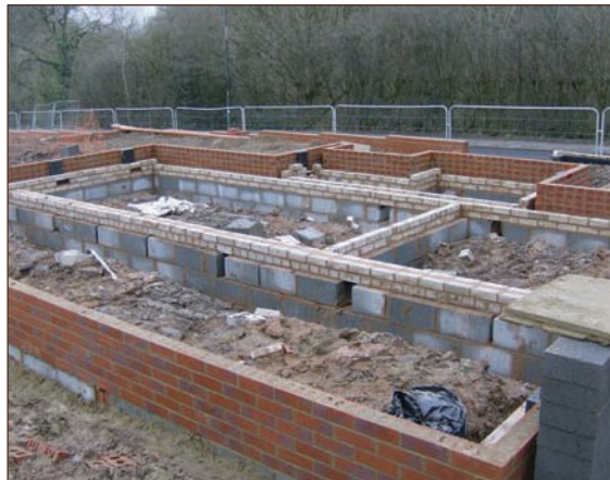
Figure A4.34 Open void >300mm deep, good ventilation through internal sleeper walls (courtesy Smith Grant)
