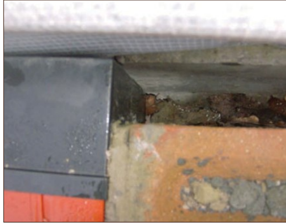
Figure A4.86 Cavity is becoming blocked with detritus. The vent holes in the beam are no longer visible (courtesy Smith Grant)
