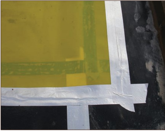
Figure A4.19 Well-constructed joints with gas resistant DPC, lap and double sided butyl joints visible beneath semi-transparent gas membrane, secondary seal with proprietary single sided tape (courtesy Smith Grant)
