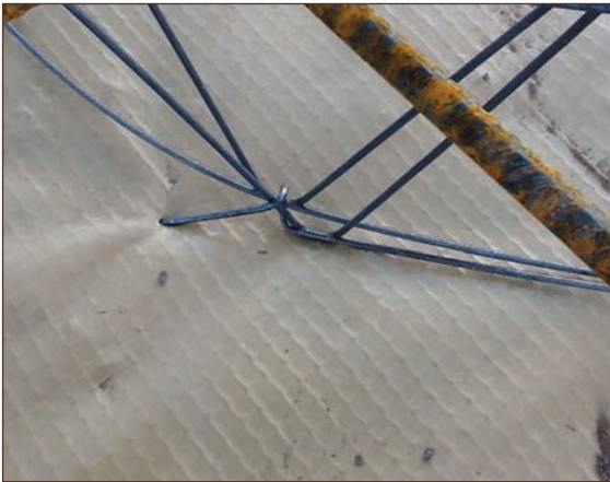
Figure A4.51 Gas membrane torn by reinforcement (courtesy MEC Environmental Ltd)
