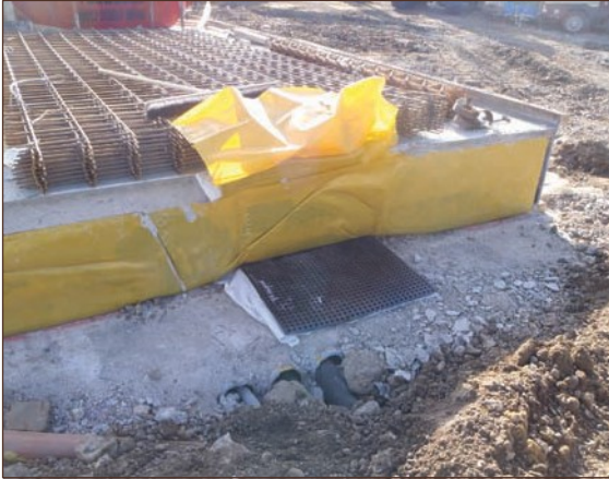
Figure A4.7 Geovent protruding out of the frontage of the unit. Gas membrane along the sides of the slab preventing lateral gas ingress (courtesy Alderburgh Group)
