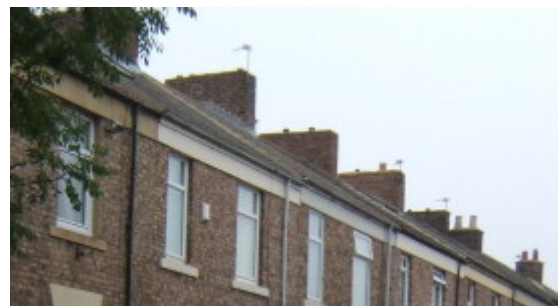
Loss of chimney pots
