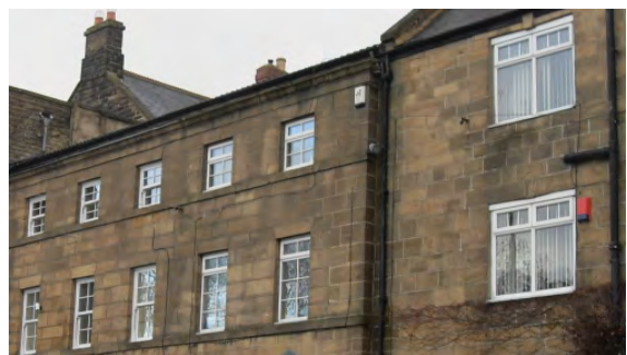
Inappropriate PVCu windows
