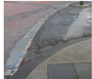
Poor quality repairs
