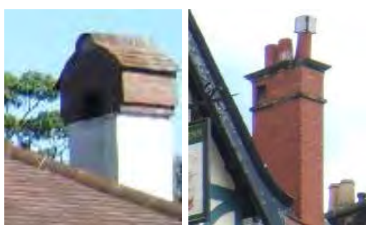
Examples of particularly interesting chimneys: 28 Northumberland Avenue, Ship Inn, East Avenue, Cheviot View, and Kyle House
