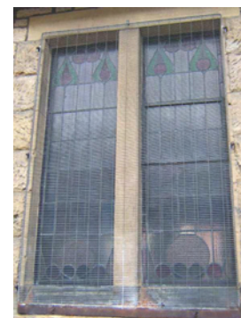
Art Noveau windows at St. Andrew's Church obscured by metal grates
