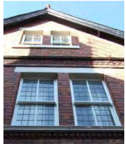
Setting window back in a reveal adds character and depth to the elevation
