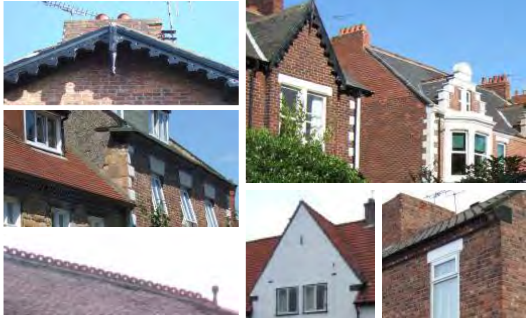
Above: Verges finished with timber bargeboards, stepped stone watertabling, and left plain. Simple brick eaves and ornate overhanging eaves. Crested ridge and terracotta finial. Below: unity to terraces comes from single-piece roofs, plus hipped corners, Coronation Cr.
