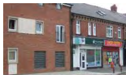
Dead frontage with no doors, Wilson Court
