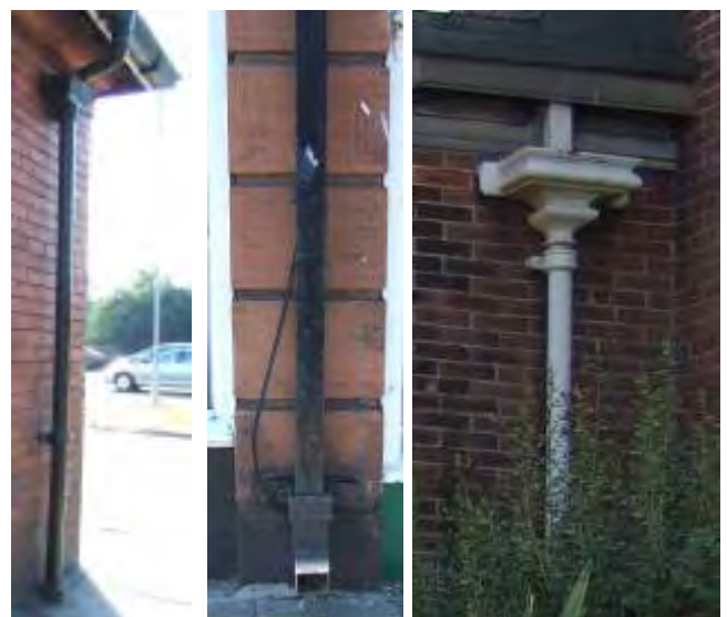
High quality rainwater goods. Station, Nos.12-40 Front St, St John's Ch.
