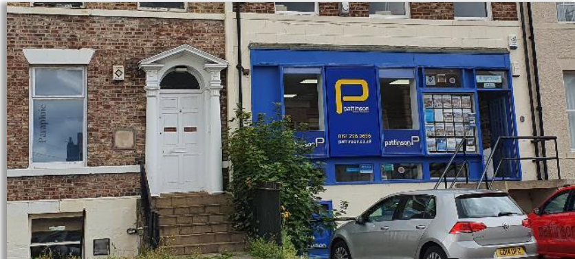
Inserted shopfront that does not respect the architecture of the building, Northumberland Place
