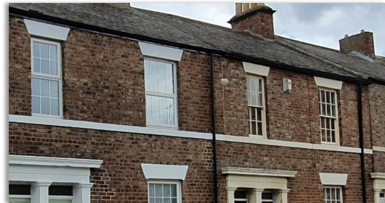
PVCu windows with flat, flimsy glazing bars and chunky frames, left, compared to traditional timber windows on the right
