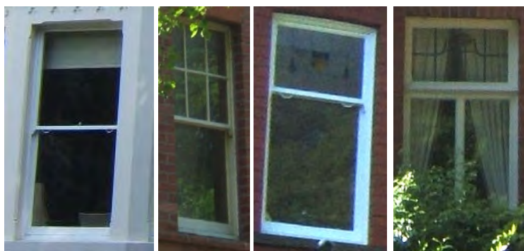
Original windows: sliding sash at Pearey House, glazing bars on top sash at The Elms, leaded sash at The Villa and leaded casement at Capel Curig
