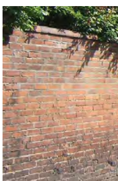
Gate pier and surviving lamp standard, left, and rear boundary brick wall, above
