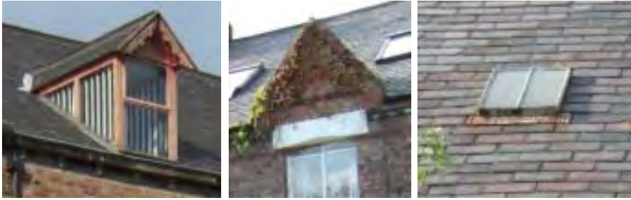
Traditional Victorian dormer, Dene Hse; peaks above 1st floor windows & early metal rooflights, Elm Tce
