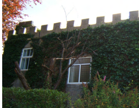
The Tower and The Gate House have flat roofs; the castellated parapet remains at The Tower
