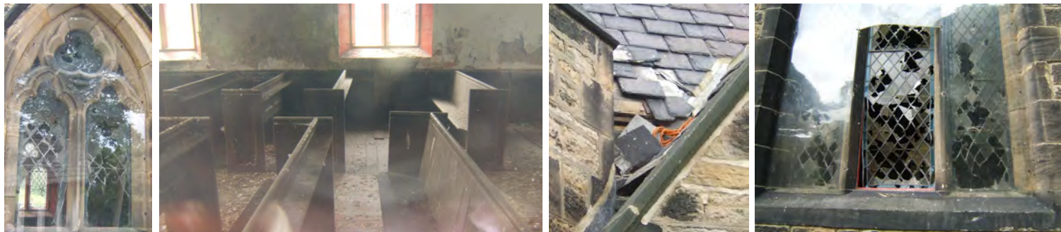
Disrepair at the Church Bank chapels, both external and internal
