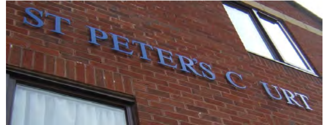
Missing letters should be replaced more quickly
